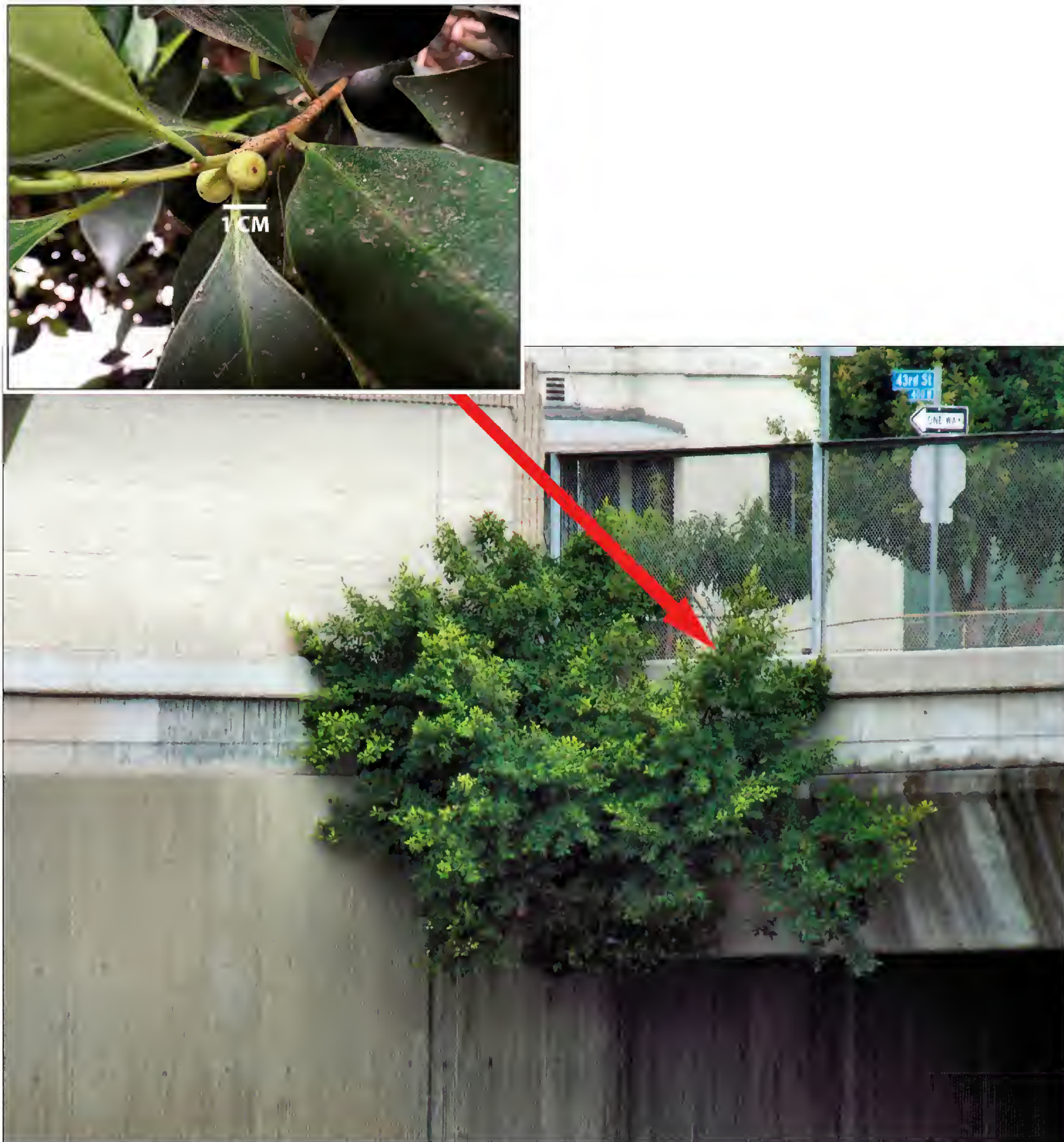
Figure 4. View of an approximately 3.2 m tall F. microcarpa tree rooted in an expansion joint of the 43 rd Street bridge on the 110 Freeway, City of Los Angeles. Note water stains on bridge and retaining wall from urban runoff, and cultivated F. microcarpa tree planted along Flower St. the in upper right-hand side of photograph. Inset photograph showing immature syconia.
